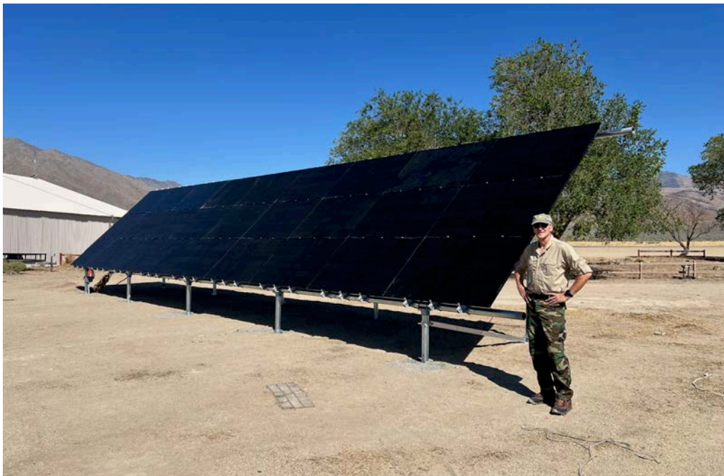
New solar array on the east side of the glider hangar
